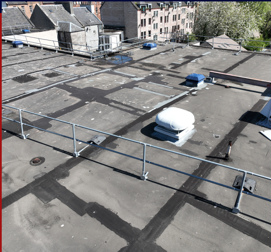
EXISTING ROOF COVERINGS WERE AGED AND WORN
