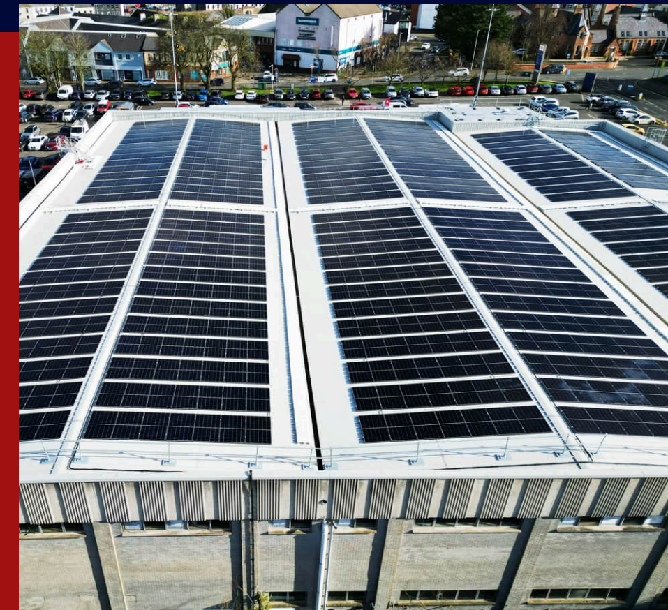
PV SYSTEM WAS CONFIGURED TO ALLOW ACCESS FOR GUTTER MAINTENANCE
