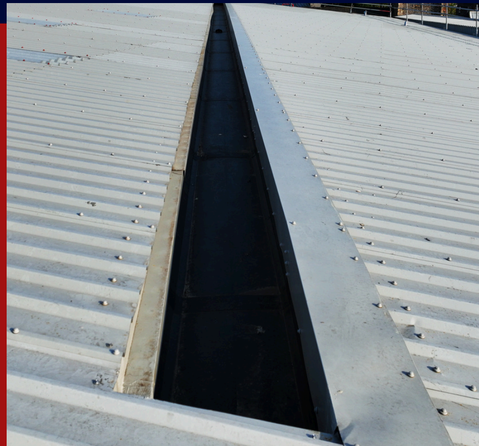
A NEW CENTRAL VALLEY LINER WAS INSTALLED UTILISING THE UNIFOLD GUTTER SYSTEM
