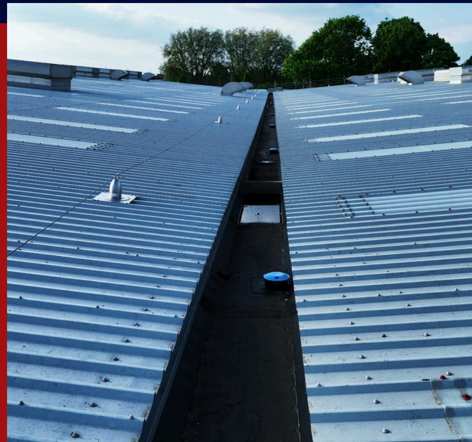
NEW CENTRAL VALLEY LINER USING UNIFOLD GUTTER SYSTEM, ALONG WITH NEW SIPHONIX.
