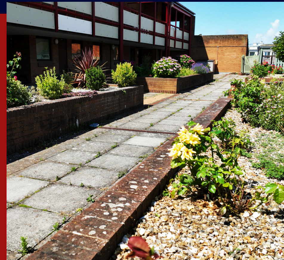
THE EXISTING SLABS AND PLANTERS WERE LOOKING TIRED.
